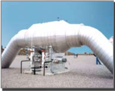
A 96" DIAMETER PEERLESS SWIRL TUBE SEPARATOR INSTALLED IN A GAS GATHERING SYSTEM. TYPICAL FLOW IS 3 BILLION STANDARD CUBIC FEET OF GAS PER DAY.
