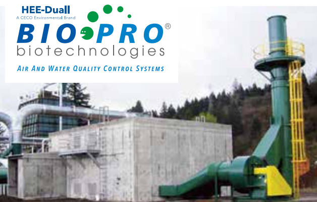
Biofilter Removing Hazardous Air Pollutants (HAPs)
