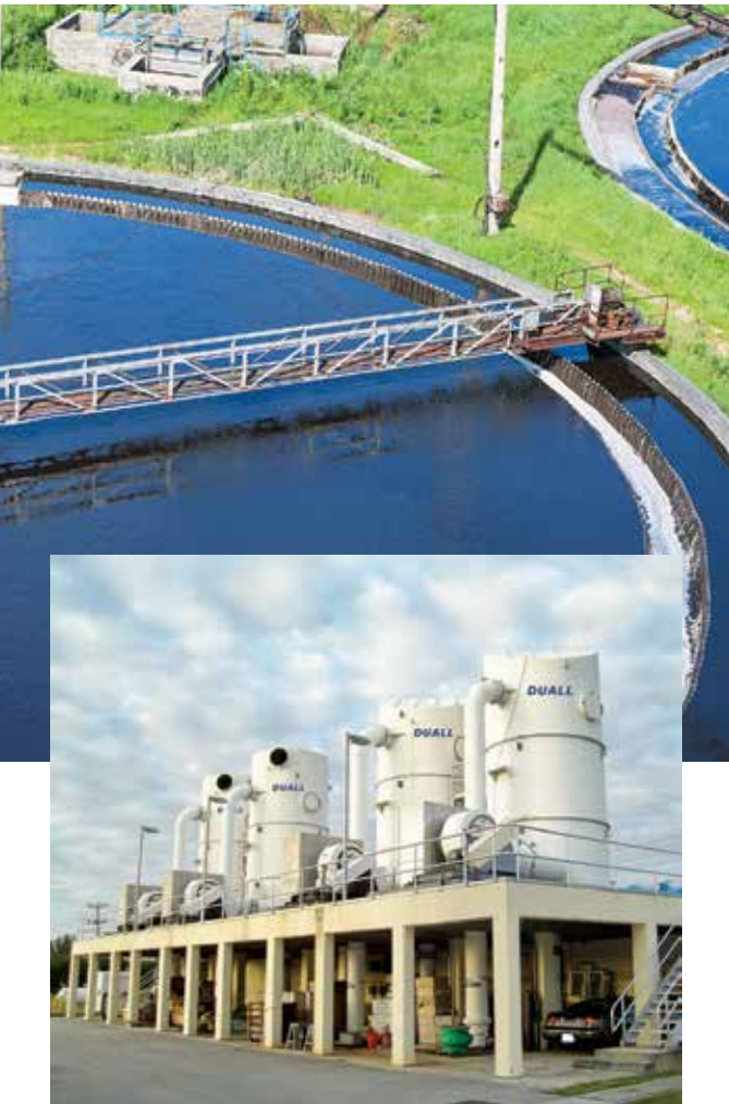
Water Production Plant with Degasifiers
