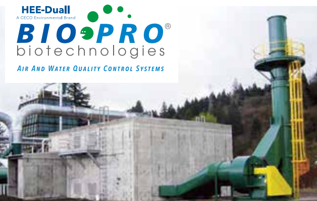
Biofilter Removing Hazardous Air Pollutants (HAPs)
