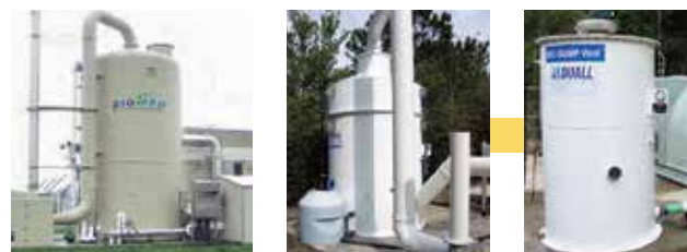
Biotrickling Filter Removing Odors
