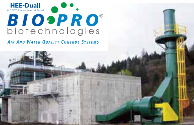
Biofilter Removing Hazardous Air Pollutants (HAPs)
