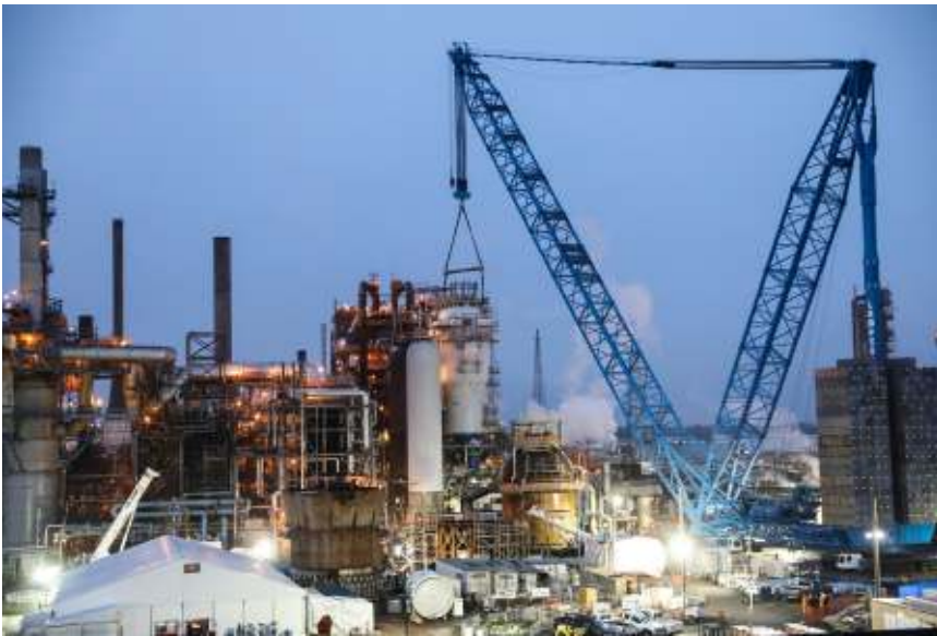
Figure 1. The FCC cyclone is lowered into the refinery. It is a key component of refinery operations and profitability. Having efficient and reliable cyclone systems is key to achieving state-of-the-art performance.
